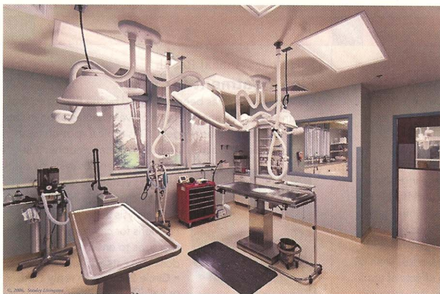
Surgery: Abundant natural light and a view of the surrounding park make this space ideal for the team. Treatment, surgery, and break areas were designed to be visually connected by large glass walls. This interior window allows a doctor to signal for an extra hand if needed.
